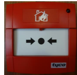
Figure 5: Fire alarm Source: CSD
