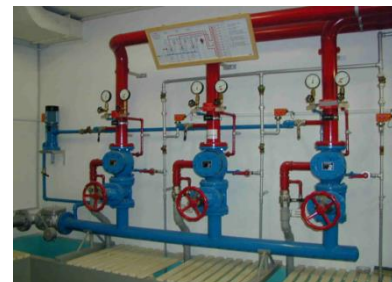
Figure 6: Sprinkler station Source: CSD
